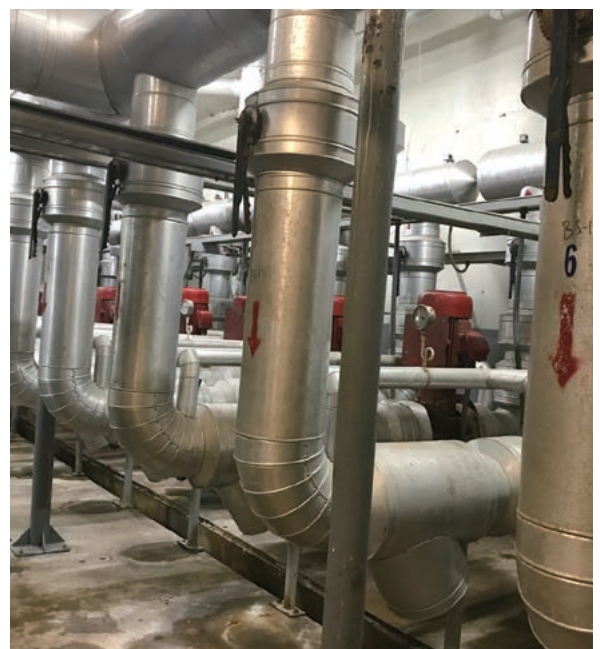
Water pipes and pumps installed in the mechanical room located below the unit.
